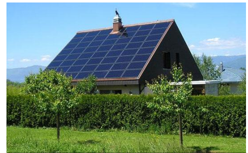
Example of a Solar Conversion System, Structure-mounted
