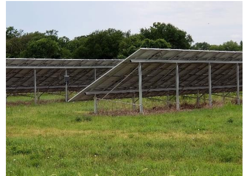
Example of a Solar Conversion System, Ground-mounted
